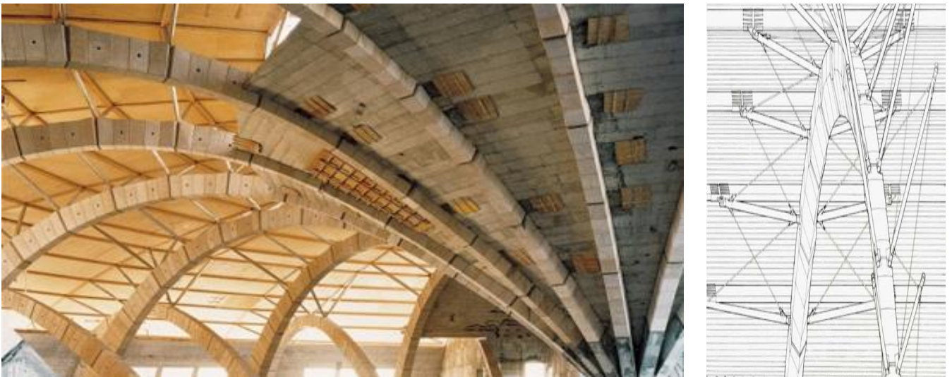
Fig. 2.9 c. Views of “Padre Pio Sanctuary” in San Giovanni Rotondo (Italy), completed in 2004 and designed by Renzo Piano. The supporting structure consists of two intermeshing rows of Apricena stone arches arranged in a circle, a total of 21, that form an inner and an outer ring with the arches of the outer ring representing scaled-down copies of the inner ones (pictures from http://www.arcspace.com/features/renzo-piano-/padre-pio-pilgrimage-church/ ).
