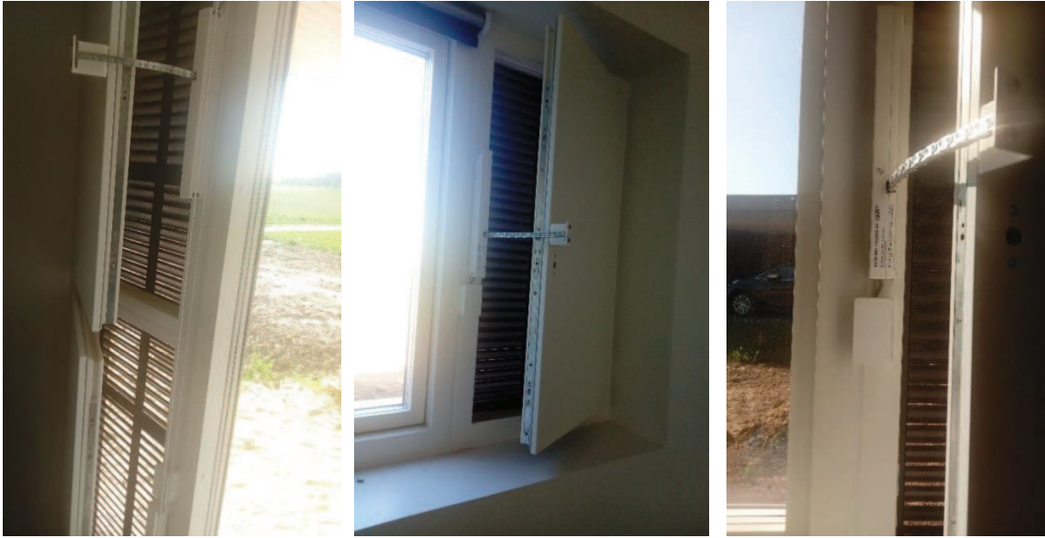
Figure 4. Details of ventilation louvers installed in the windows.
