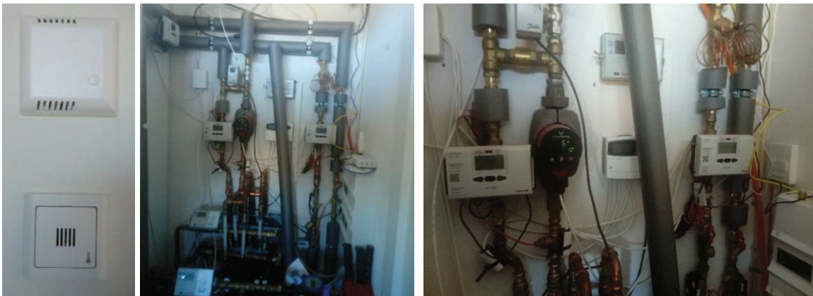
Figure 5 - Indoor air quality sensors (CO 2 , temperature and relative humidity), and control system in the technical room.
