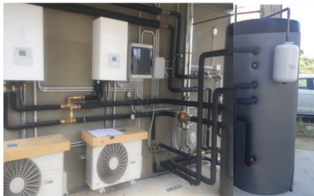
Fig. 1- The demonstrative plant installed at the DOMUS research center of the University of Calabria
