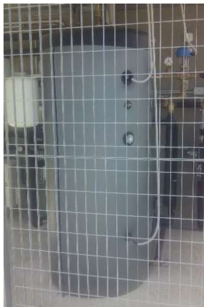
Fig. 41 – Water tank used as thermal storage system
