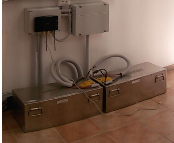
Fig. 40 – Battery storage system
