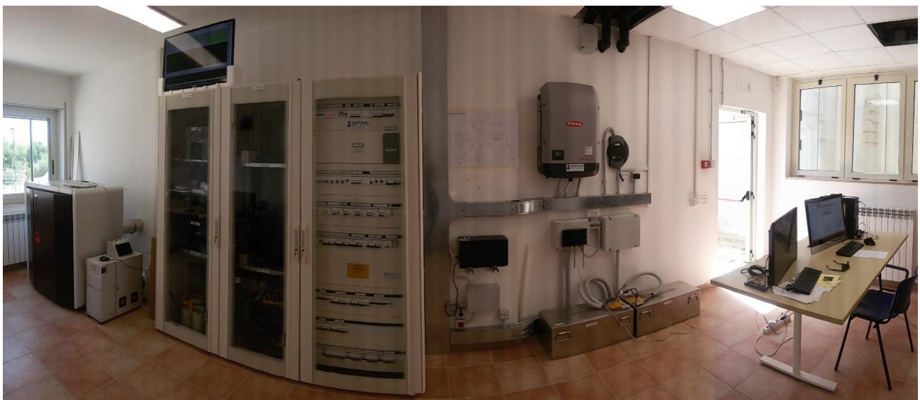
Fig. 5-5 The setup inside the building of the University of Calabria
