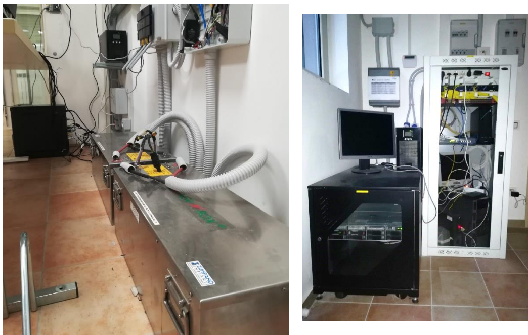
Fig. 5-7 Battery storage system (left) and critical loads (right)
