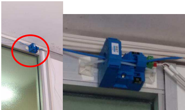
Figure 4.15 Instrument used to measure the electric power, AC transformer 0..50A #57645
