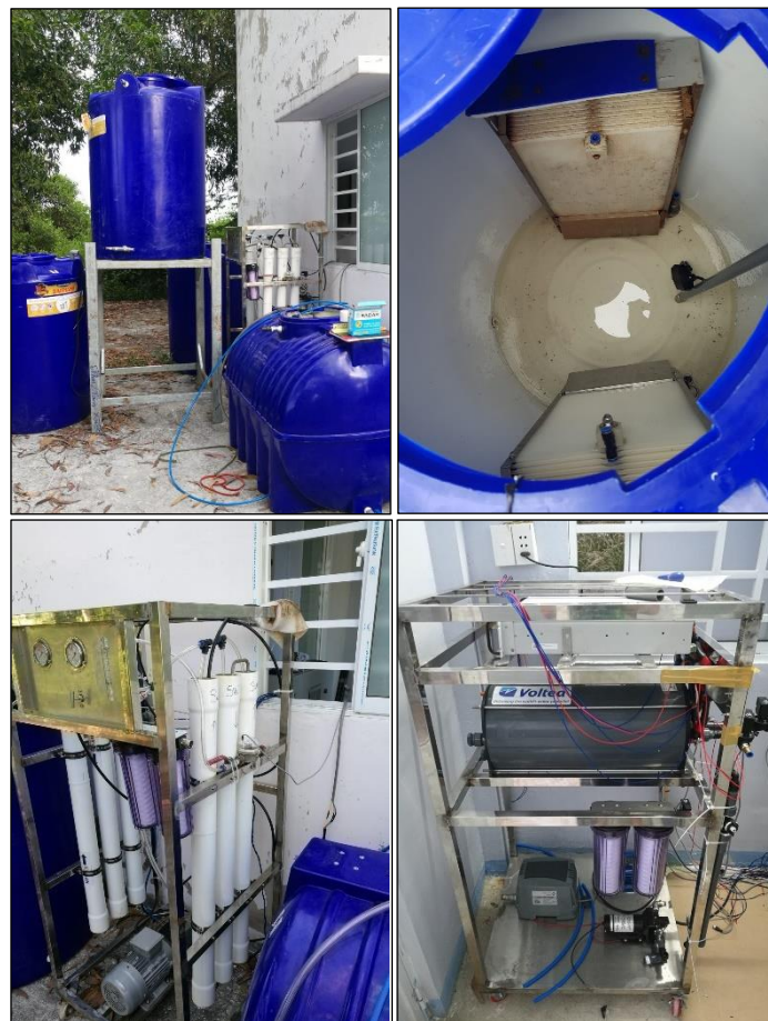
Figure 3.4-3 Pilot-scale plant LPRO+MCDI in Can Gio: a) storage tanks, b) UF pre-treatment, c) RO system and d) MCDI electrode module incl. power supply.
