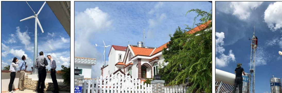
Figure 3.3-6 Wind turbine (left) and weather station installation (right) at pilot site location (centre).
