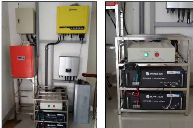
Figure 3.3-5 Inverter, batteries, charge controller (load dump) and utility meter.
