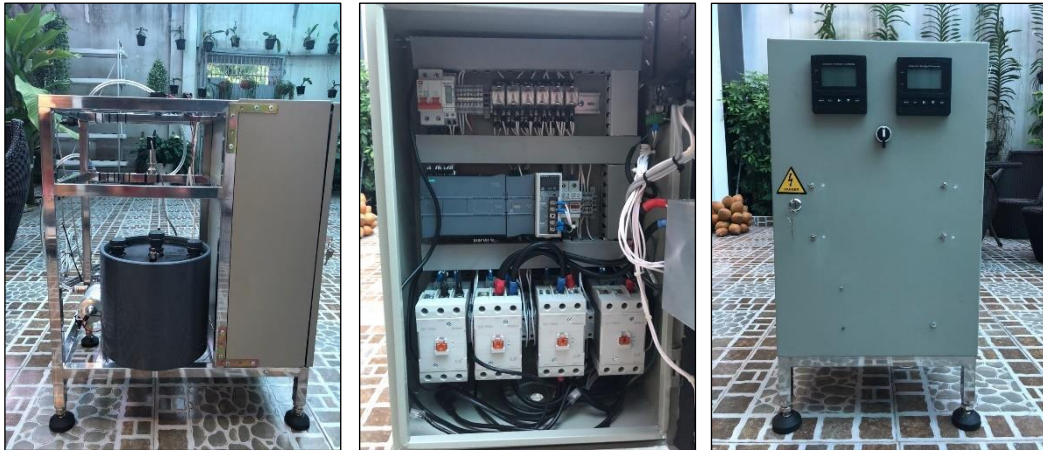
Figure 3.3-3 MCDI pilot plant for desalination including electrode module (C3, Voltea®) (left), electric cabinet (center) and power supply (XP Power HDS 1500 PSI2) (right).
