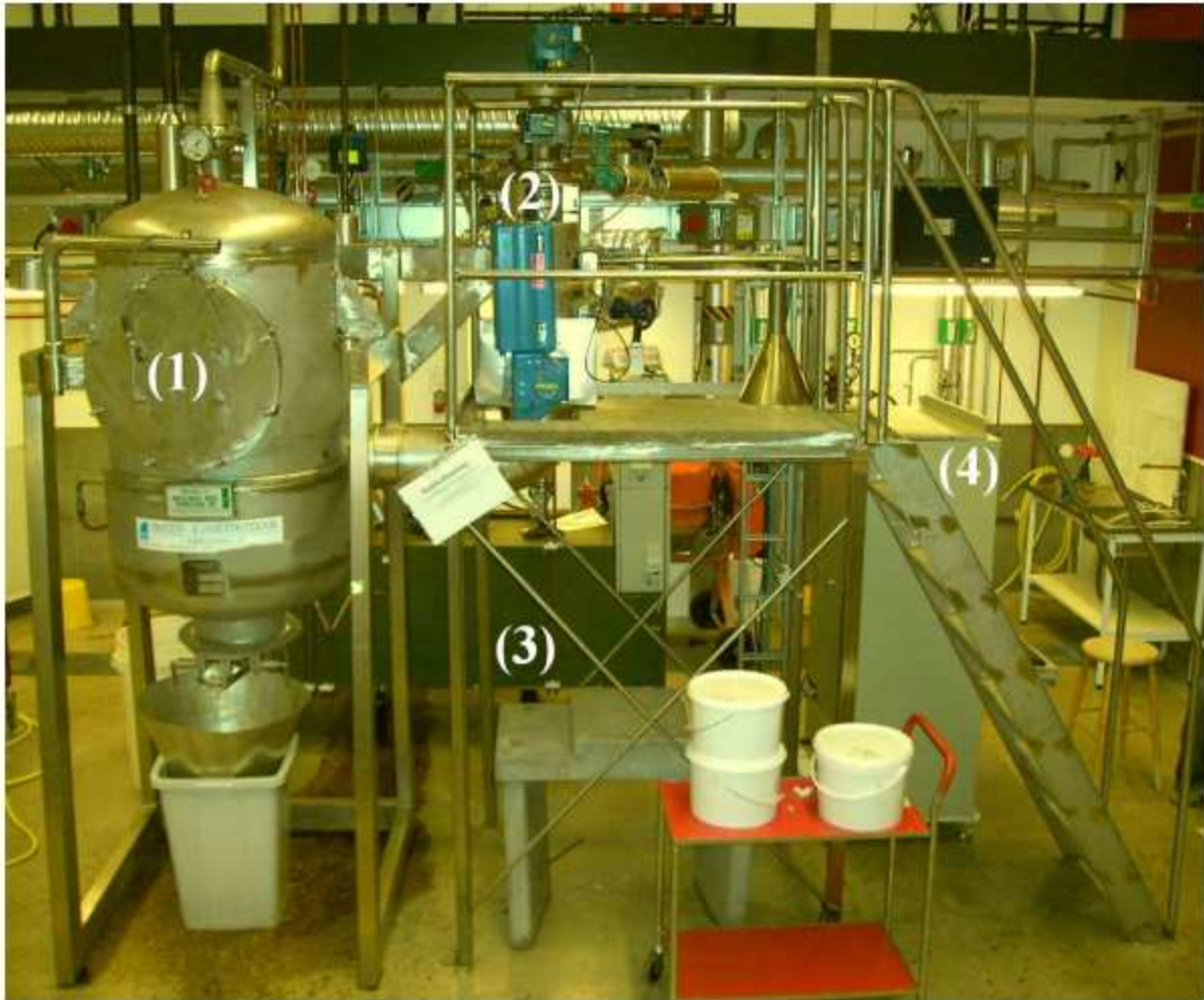
Fig. 4.6 Steam pretreatment unit; 1:flash cyclone, 2: reactor, 3:steam generator, 4:operator computer
