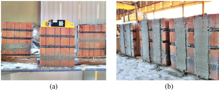
Fig. 5.10: Preparation of masonry specimens for tensile tests: (a) repair of the tested samples; and (b) strengthening of the tested samples.
