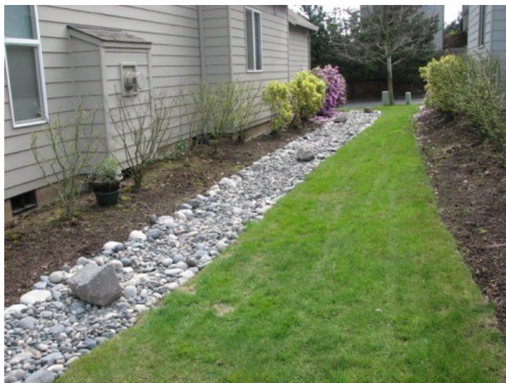
Figure 1.3 Infiltration trenches ( www.marshalls.co.uk/watermanagement )
