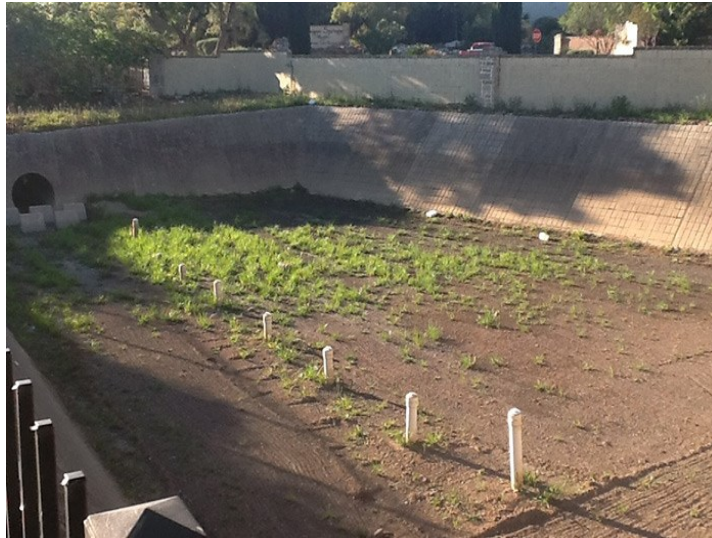
Figure 1.5 Constructed sand filter ( www.storm-tex.com )
