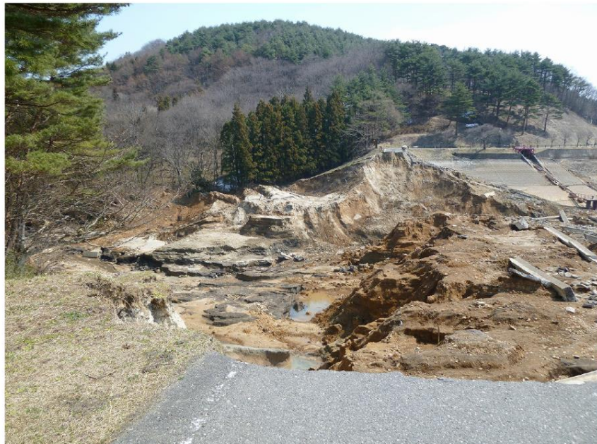
Figure 2.18: Fujinuma-Ike dam after the 2011 Tohoku earthquake (Matsumoto et al., 2011).
