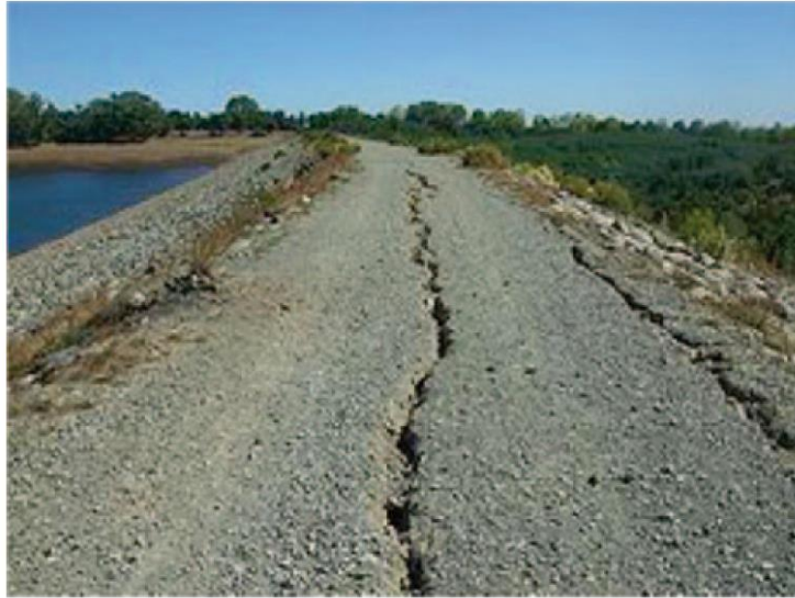
Figure 2.11: Longitudinal crack observed in Coihueco dam (from Séco and Pinto, 2015).
