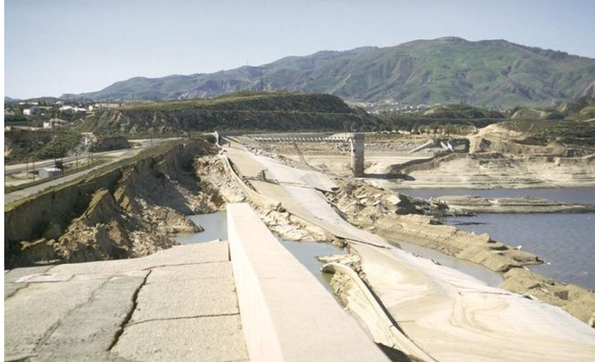
Figure 2.17: Lower San Fernando dam after the 1971 San Fernando earthquake (from Boulanger et al., 2015).
