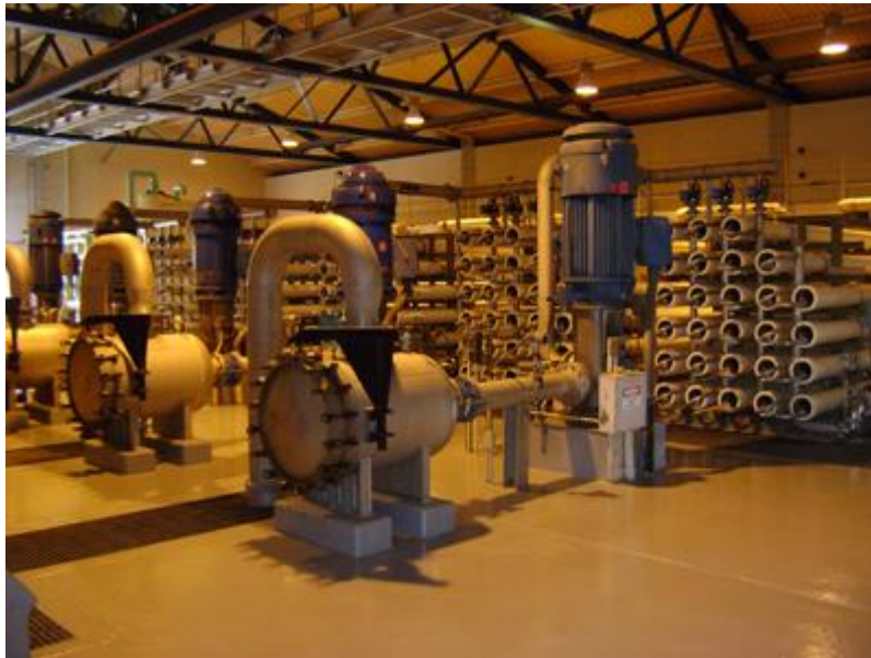
Figure 1.4 Existing RO Plant [8]
