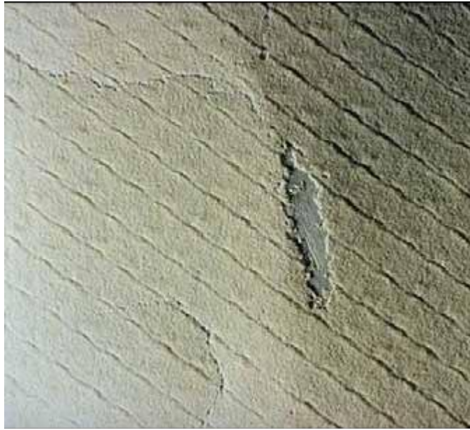
Figure 3.4 Scaling on membrane surface
