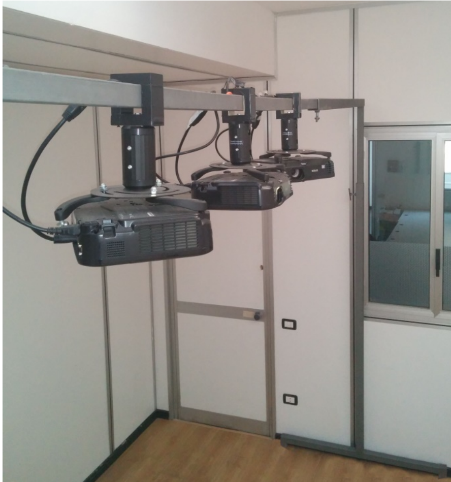
Figure 5.10: View of the projectors installed on the structure
