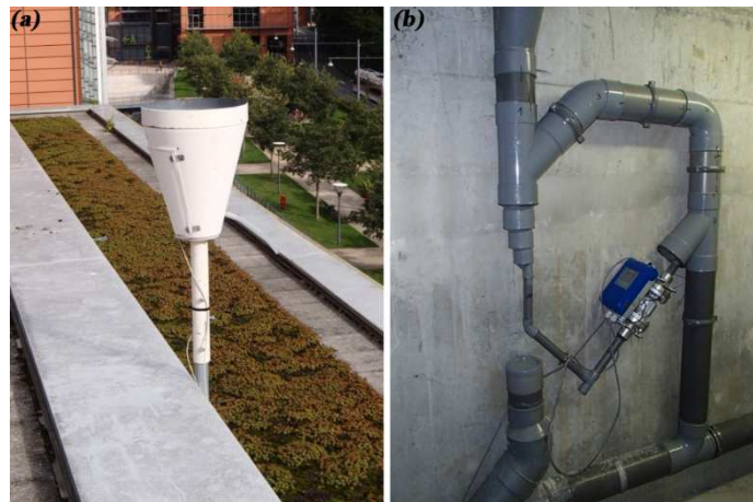
Figure 4.5. Monitoring of the Lyon Congress Centre green roof. Left: rain gauge; right:magnetic flow meter (photos LGCIE-DEEP).
