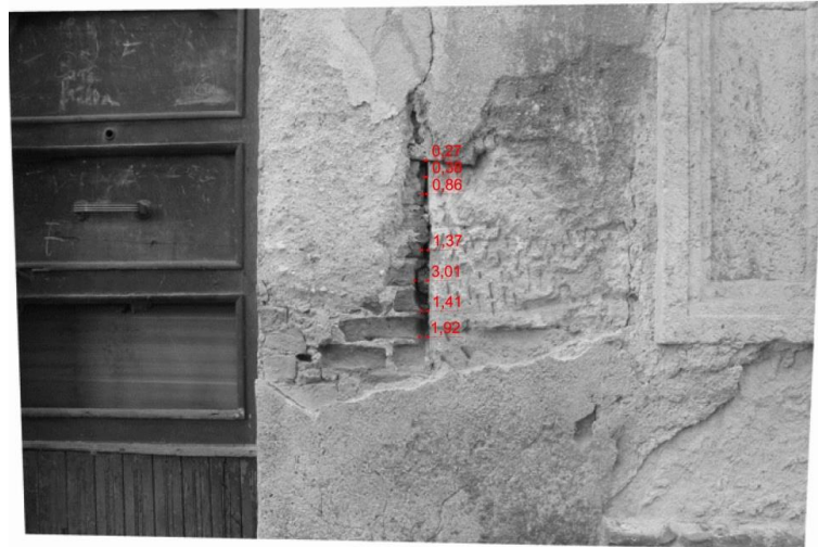
Figure 2.3: Rectified image of a crack.
