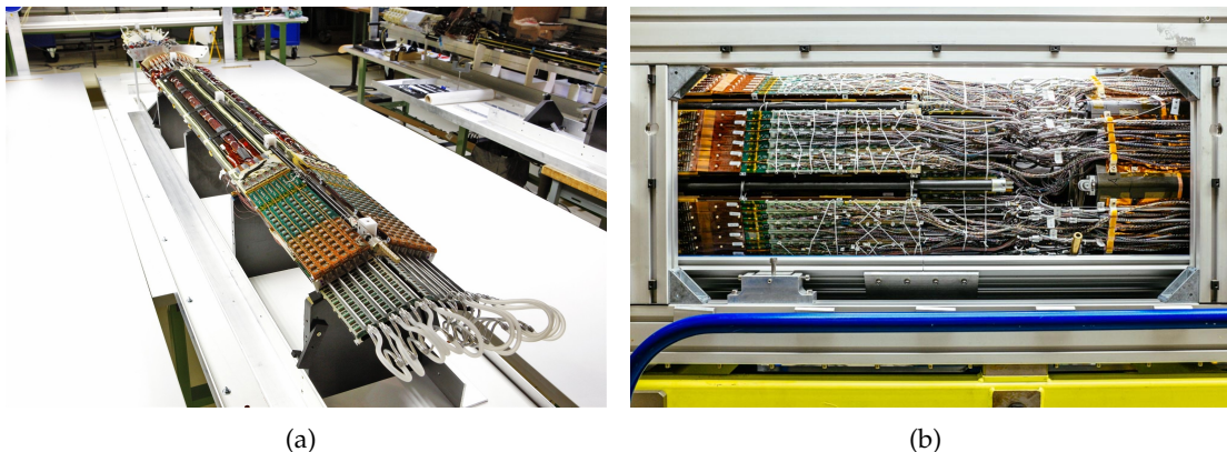
FIGURE 2.18: (a) A quadrant of the bare new Service Quarter Panel (nSQP). The front side is connected to the detector. (b) Pixel services after re-assembly in LS1. In this photograph, the right-hand-side is the detector, and the left-hand-side represents the services. Ref. [72].
