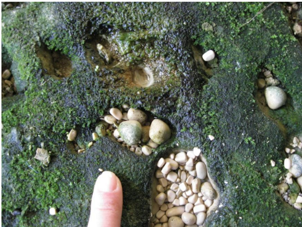
Fig. 4.21. Top of the reinforced concrete base on which occur sub-spherical “cave pearls”.
