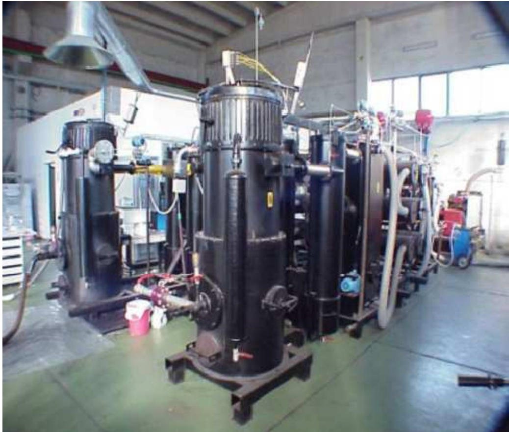
Figure 3.4: DownDraft fixed bed gasification plant.
