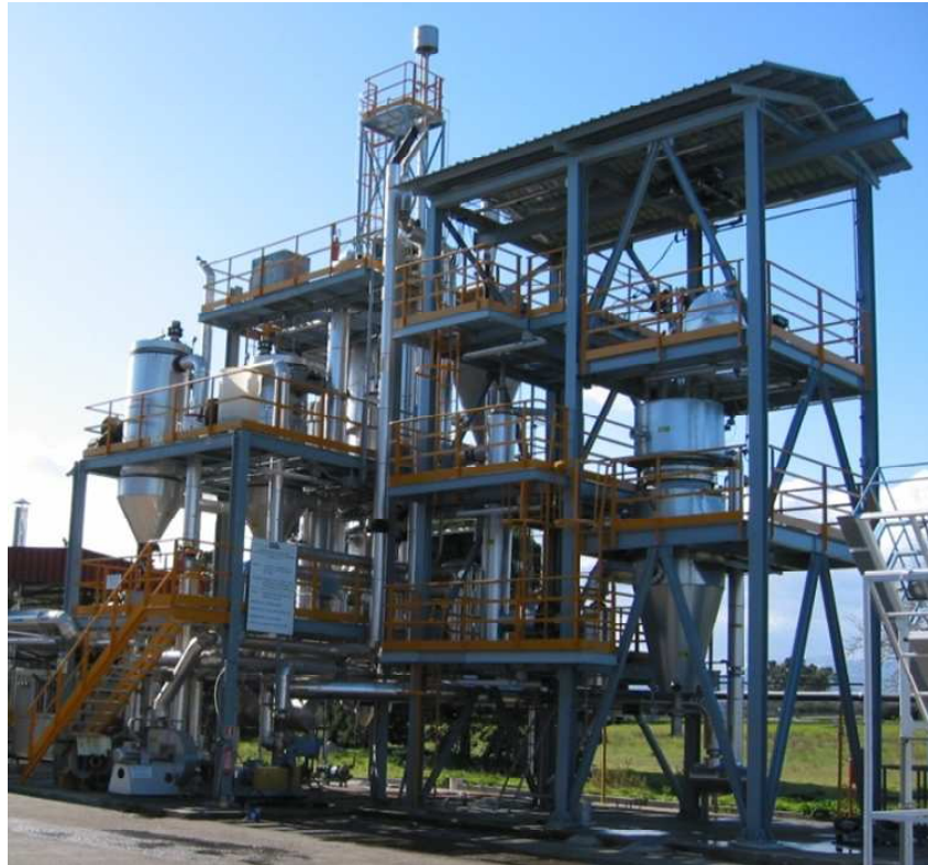
Figure 3.1: the 500 kWth gasification plant.
